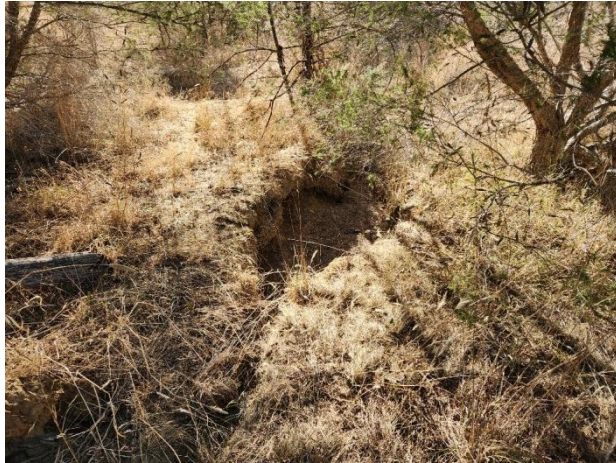
Tunnel erosion on reach banks
