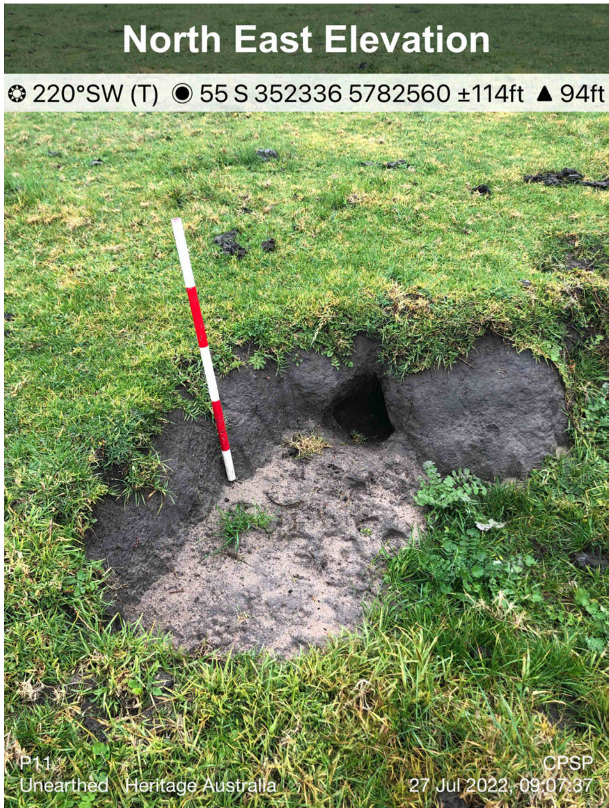
Figure 5-1 Example of small, localised exposure around rabbit burrow in VPA Lot Number 11 (GSV averaging 5%)_MSteel_27July2022
