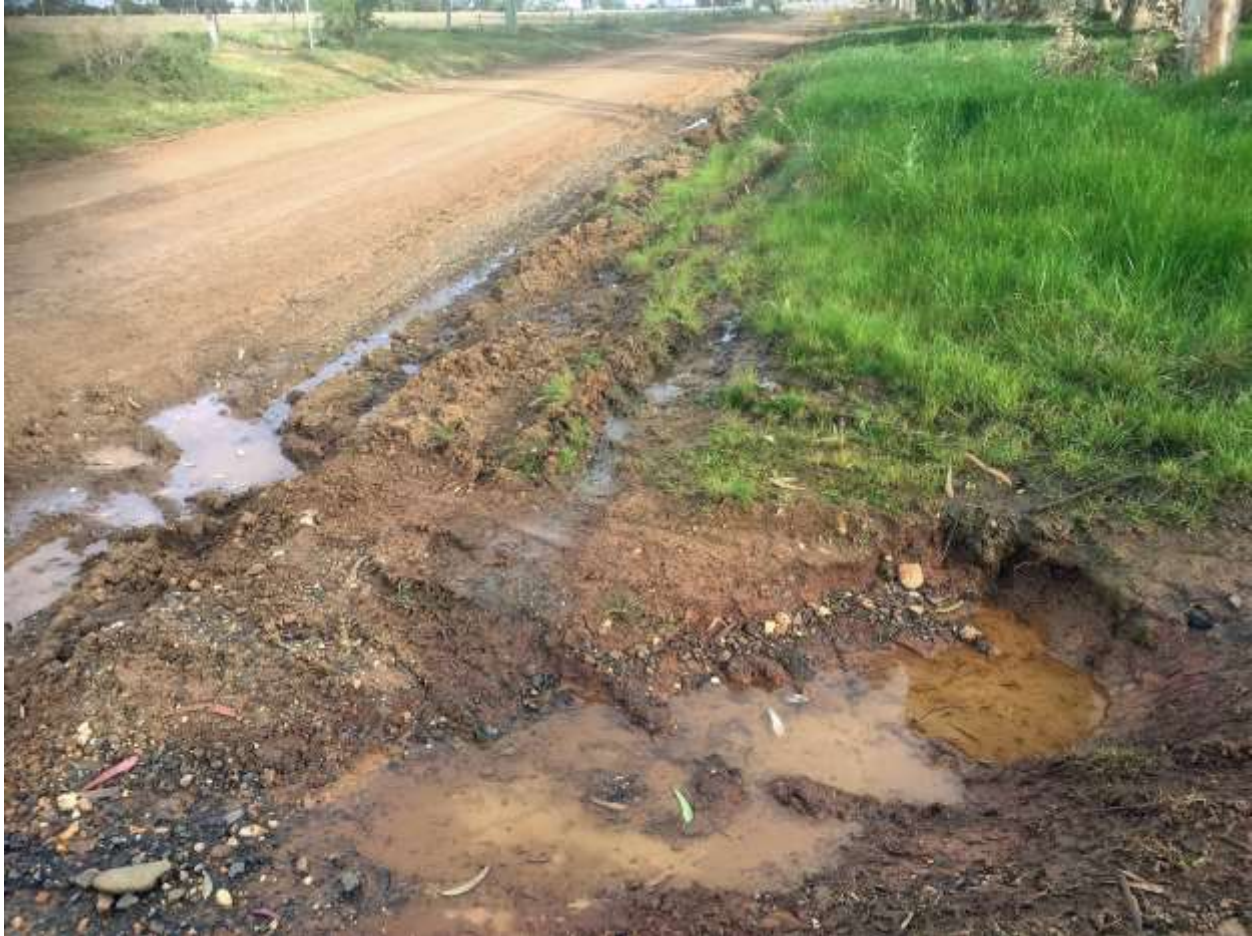
Photograph 11 Erosion scour on the western side of Paynes Road caused by storm water runoff. This erosion is the result of poor water management and is causing excessive amounts of sediment to be washed into the wetland.
